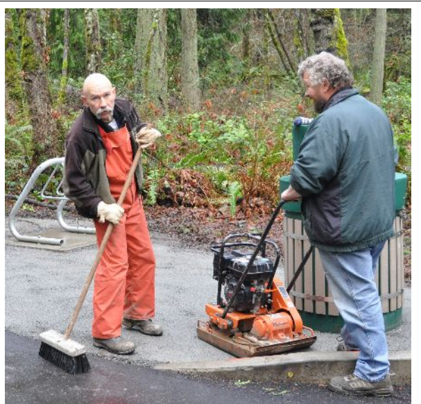
Saanich crews put the finishing touches on the new parking lot area. A job well done!
