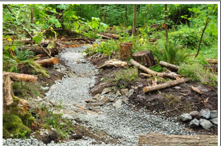
Tributary 3 after clearing and gravel bed placement. Subsequently, natural vegetation was planted along the banks.
