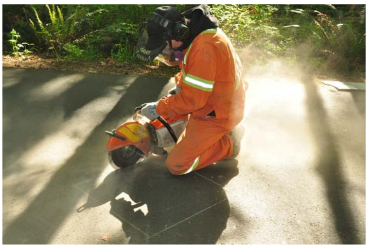
Cutting asphalt for installation of distance and altitude marker stones. Engraved stones were placed every 250m along the walk up the “Churchill Challenge”.
