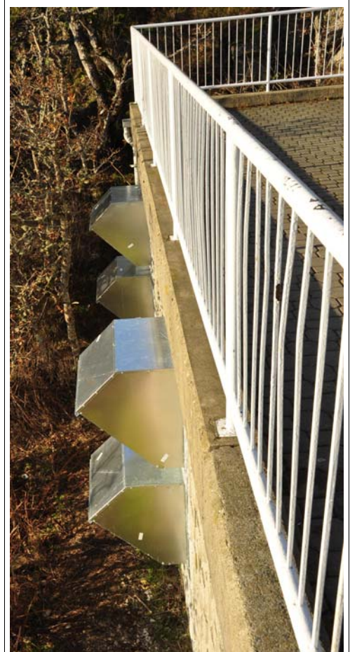
Four of six new vent covers at the transmitter building.
