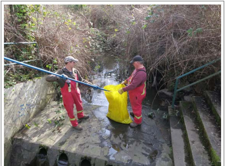
Saanich Crews respond to a hotline phone call reporting a possible spill.
