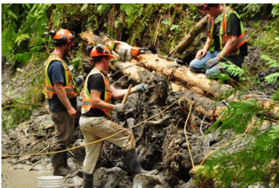
Any logs not securely cabled will be washed out with the first storm surge!
