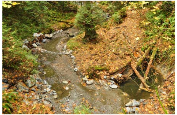
View from Ash Road. Creek was widened to slow water. Banks were armoured with boulders to prevent further erosion.
