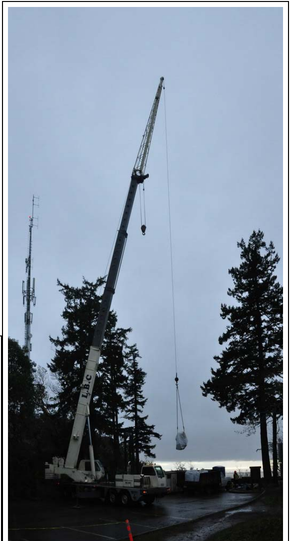
Crane used to remove old tower debris and lift top soil to summit.
