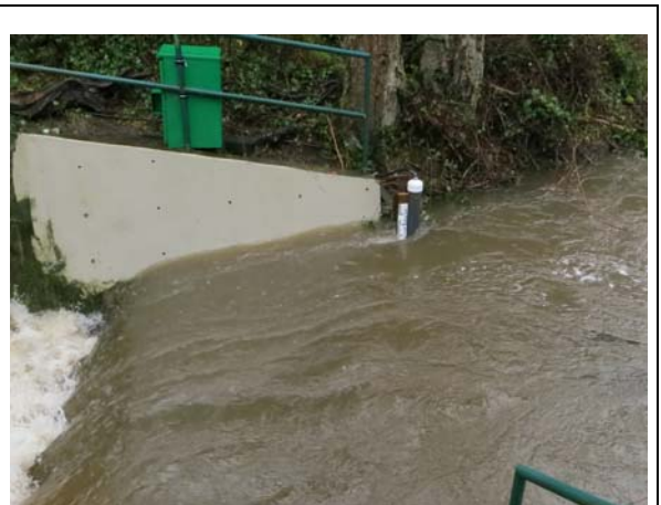
Storm surge at the weir. The scale shows the depth is 40cm above the top of the weir.
