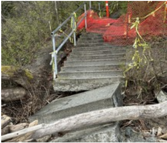
Old stairs undermined by creek high flows
