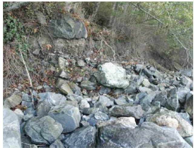
"Failure of the rip-rap revetment has allowed continued erosion of the shoreline."[WSP Canada Inc.]
